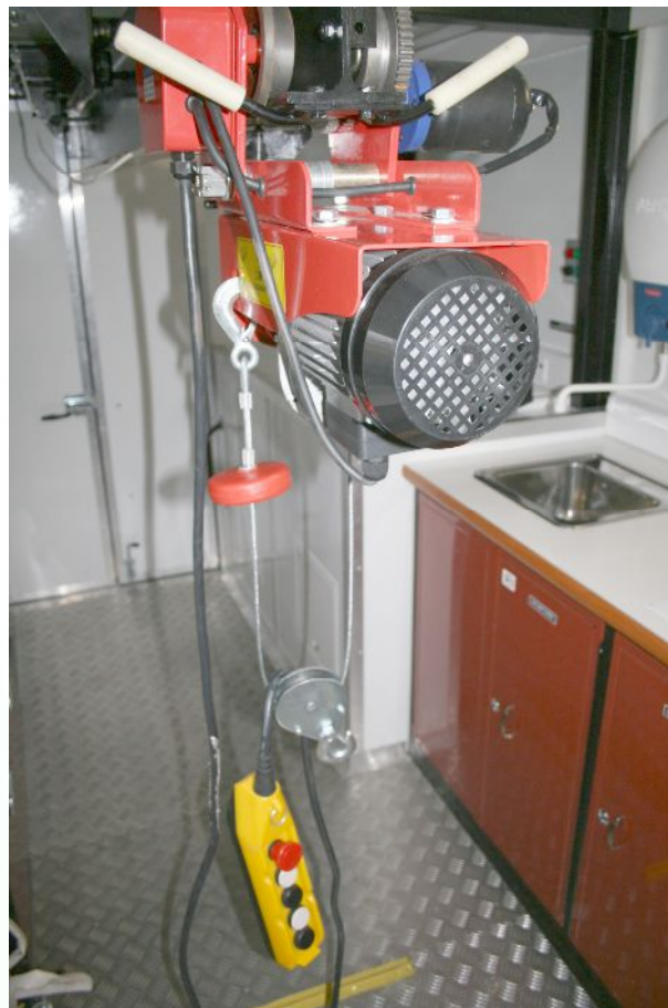
Photo 9,10 – General view on the load lifting device
