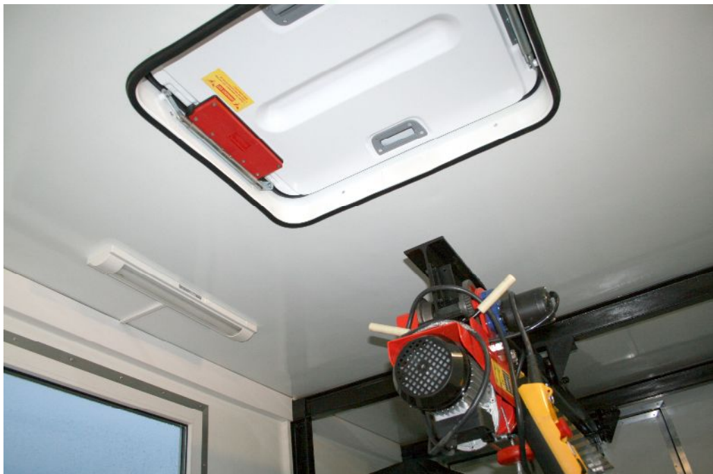
Photo 8 – View on the organization of the emergency conditioning and load lifting device view
