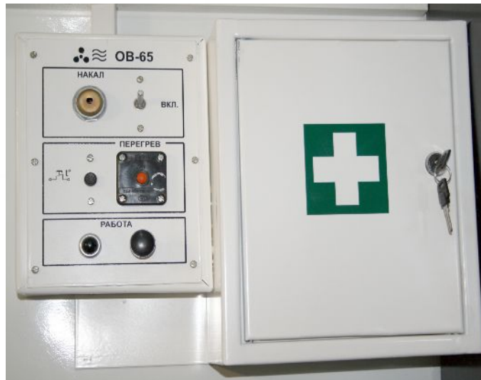
Photo 12 – General view on the heating control switchboard
